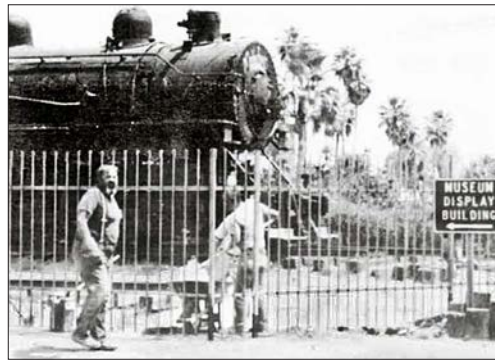
At left, Ron Schofield welding up a section of fence, and at right Ron, Steve Blais, and Tom Houser pouring cement for the fence posts. from The Chandler Branch, May 1989
